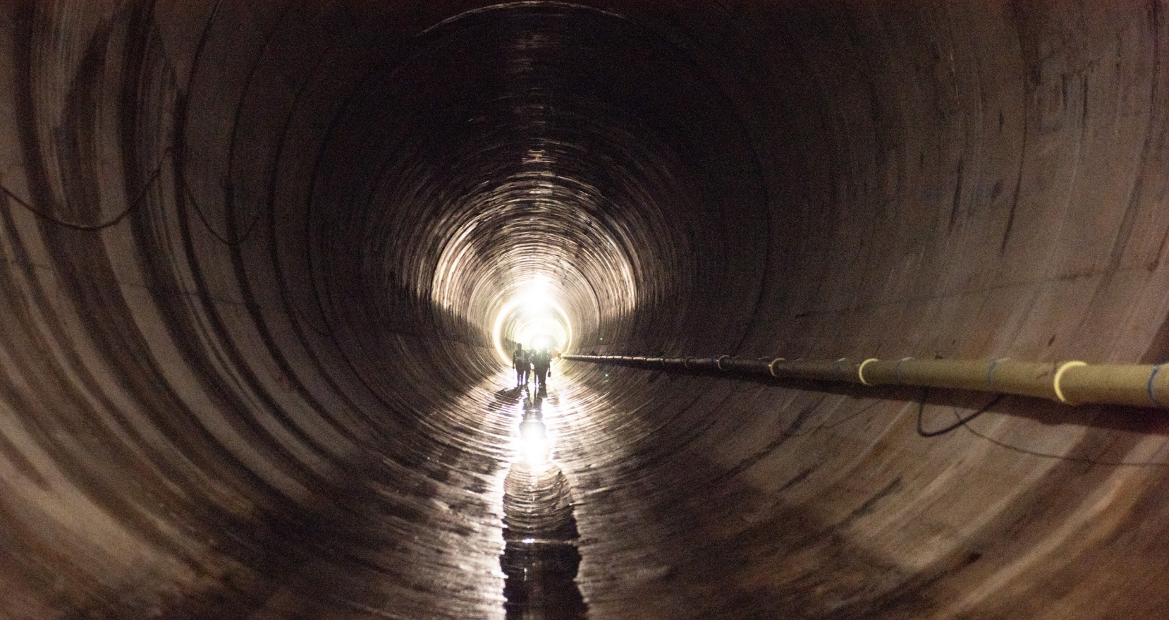
Workers examine the inside of the Des Plaines Inflow Tunnel, part of the MWRD's Tunnel and Reservoir Plan.
