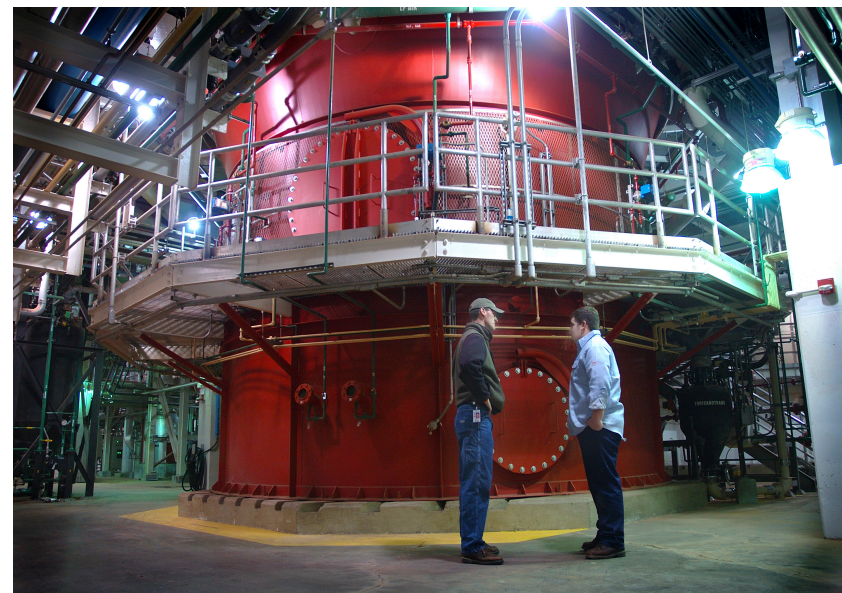
Wastewater solids (SSI) incinerator, St. Paul, MN
