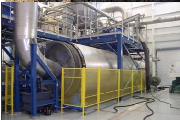
Rotary drum dryer, South Cary, NC
