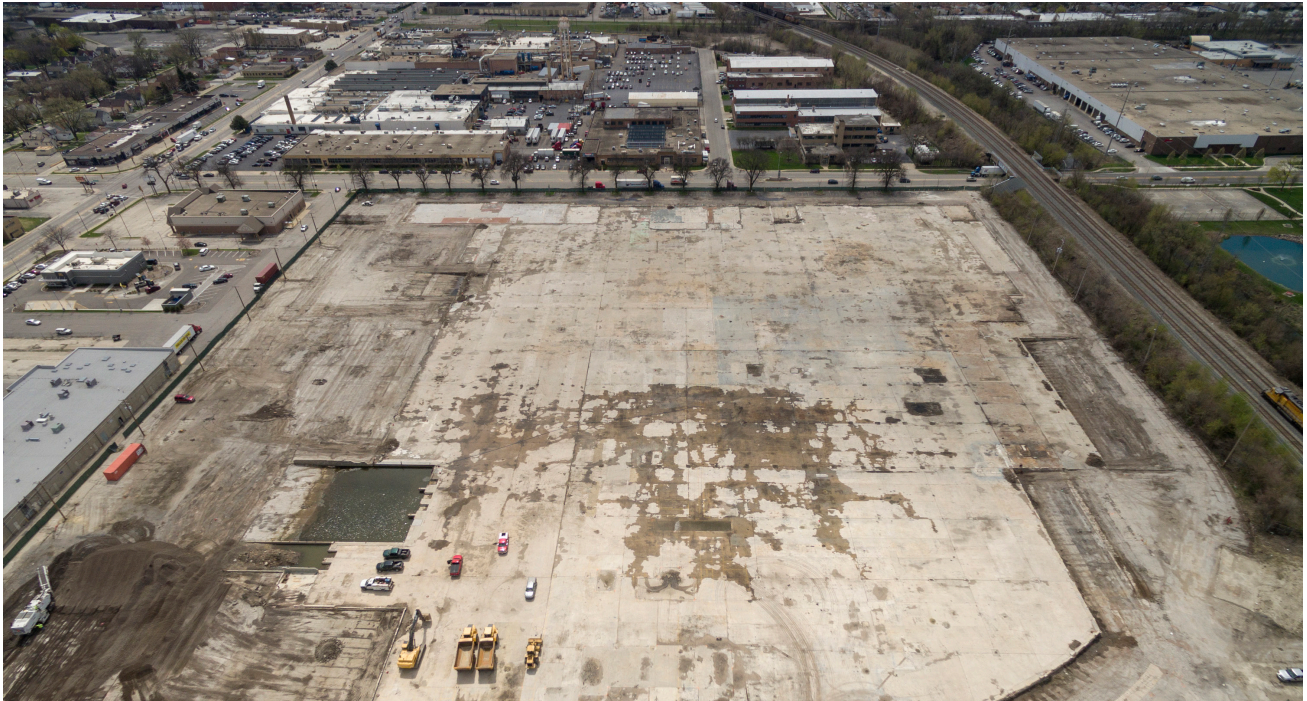
Ground was broken on the Addison Creek Reservoir, in Bellwood, Illinois, in 2019. When completed in 2023, it will be able to hold close to 200 million gallons of stormwater.
