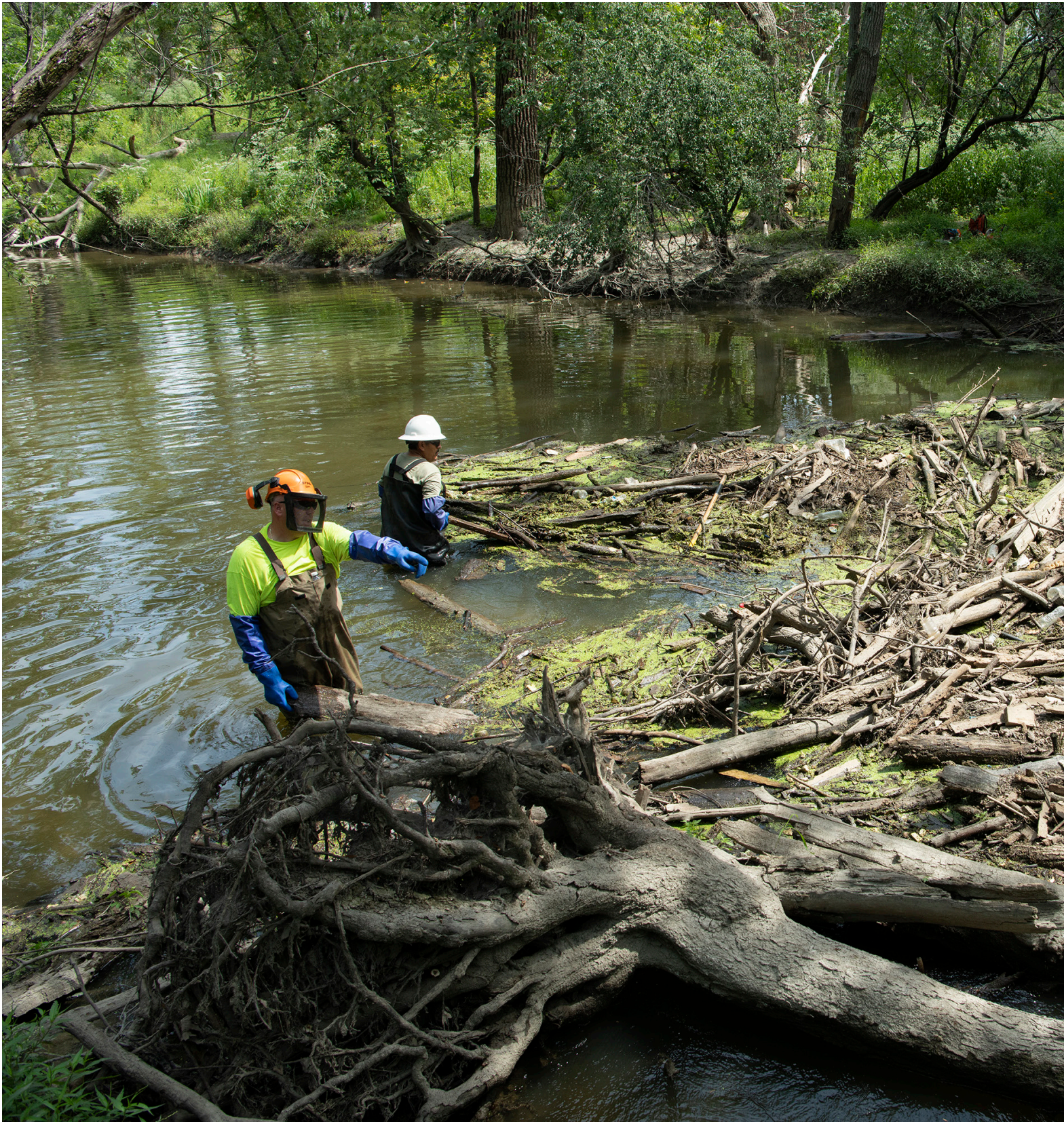
As part of the MWRD Small Streams Maintenance Program (SSMP), a crew works to remove a blockage of tree limbs in the North Branch of the Chicago River near Miami Woods and Prairie in the Forest Preserves of Cook County. This critical work reduces flooding and keeps the river flowing.
