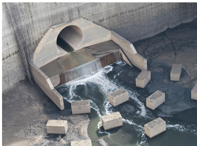
At the headwall and apron of the tunnel connection of the McCook Reservoir, concrete blocks withstand the force of the water emanating from the tunnel and prevent erosion of the reservoir floor.
