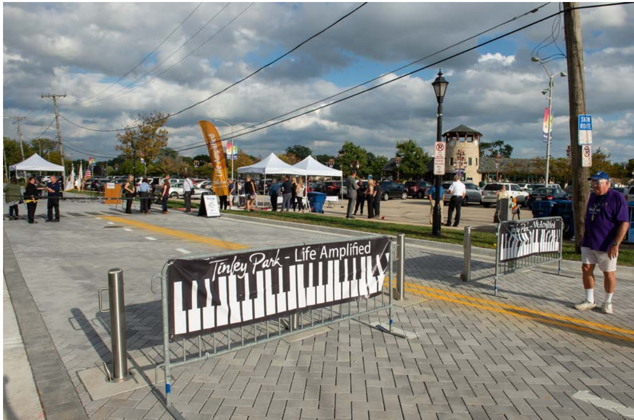
A new permeable paver project on North Street in Tinley Park was unveiled by MWRD Commissioners Debra Shore and Kim Du Bucllet along with Tinley Park officials in October as part of the Harmony Square development near the Metra Station. The MWRD contributed $200,000 to replace asphalt with 16,500 square feet of permeable pavers on North Street, which will provide more than 69,000 gallons of stormwater storage on site.
