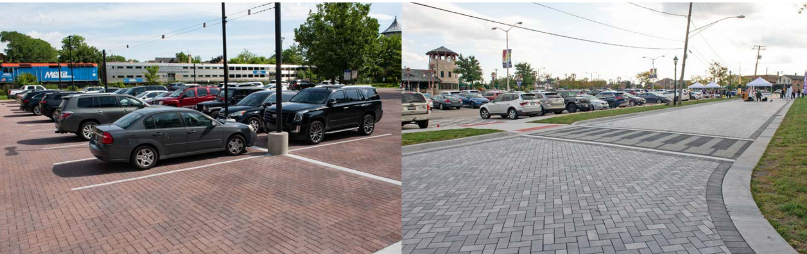
▲ Permeable pavement in Riverside Metra parking lot (L) and Tinley Park (R).
