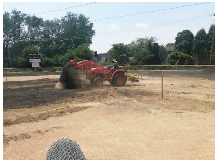
Tractor with bucket attachment for application of heavy rate of biosolids to restore ball fields.
