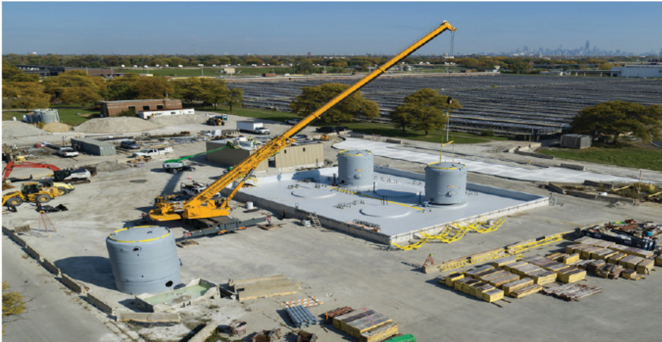
Construction of the chemical addition backup system showing placement of the chemical storage tanks at the Stickney Water Reclamation Plant.
