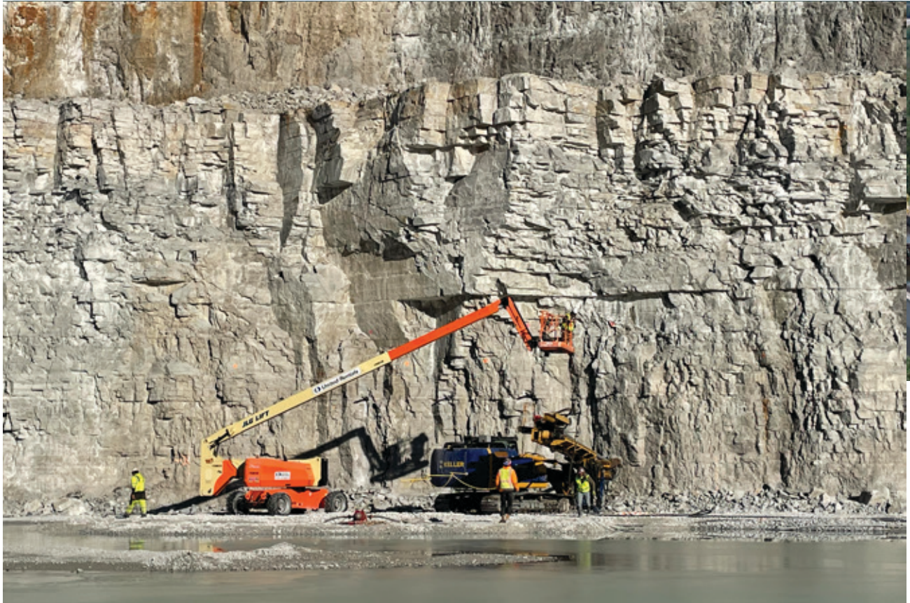
Installation of rock anchors on the rock wall at the Thornton Rock Dam.
