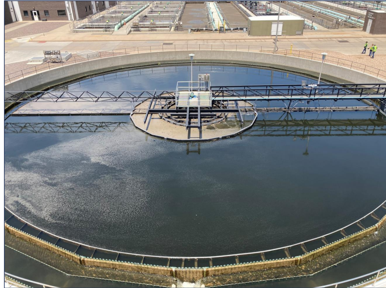
DAS Pilot Secondary Clarifier
